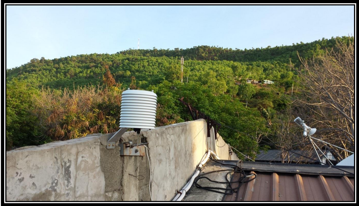
Figure 3. EnviroLINK installed on top of the conference building. Dili hills are in the background.
